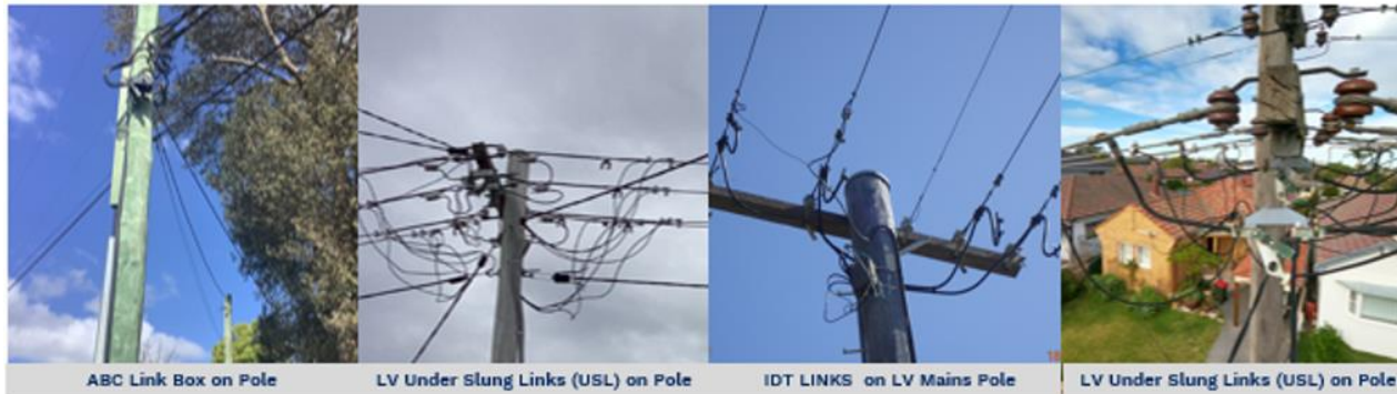
Image of Low voltage links
