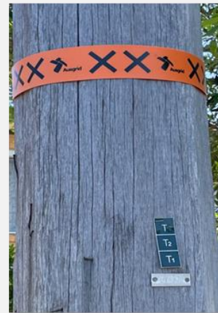
Image of Defective pole marking – Orange Band
