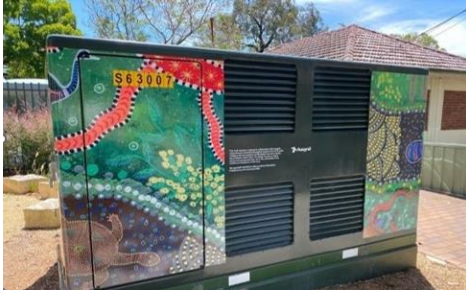
Image of Kiosk substation
