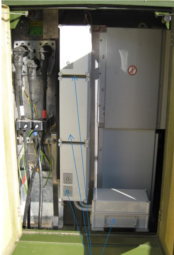
WTC DMC arrangement of Powersense boxes
