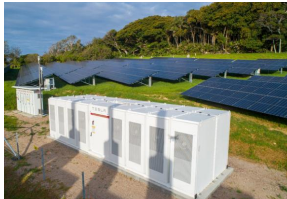
Lord Howe Island Microgrid
