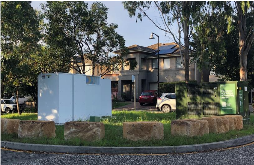
Bankstown Battery successfully commissioned on 27 May 2022. Noise testing continuing through to end of June.
