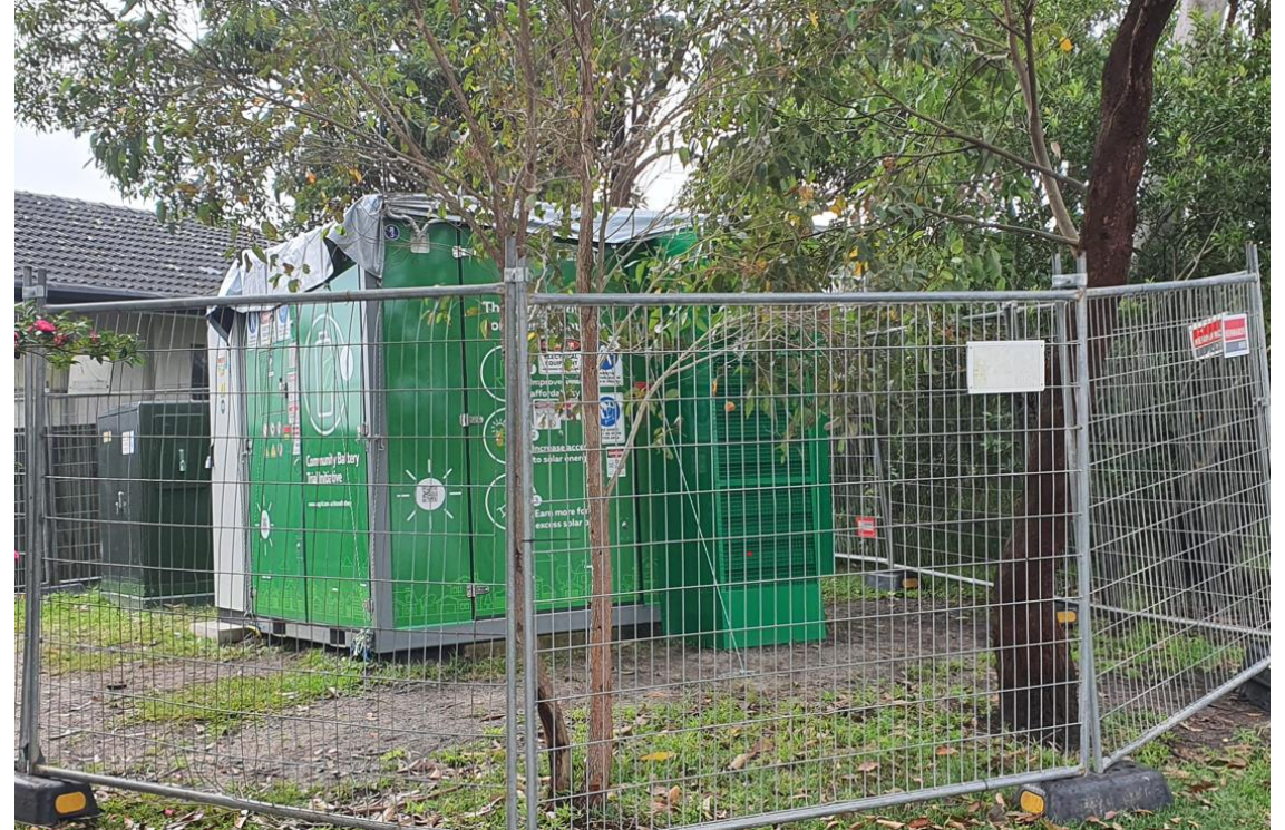
Beacon Hill battery trapped and fenced off due to water ingress.
