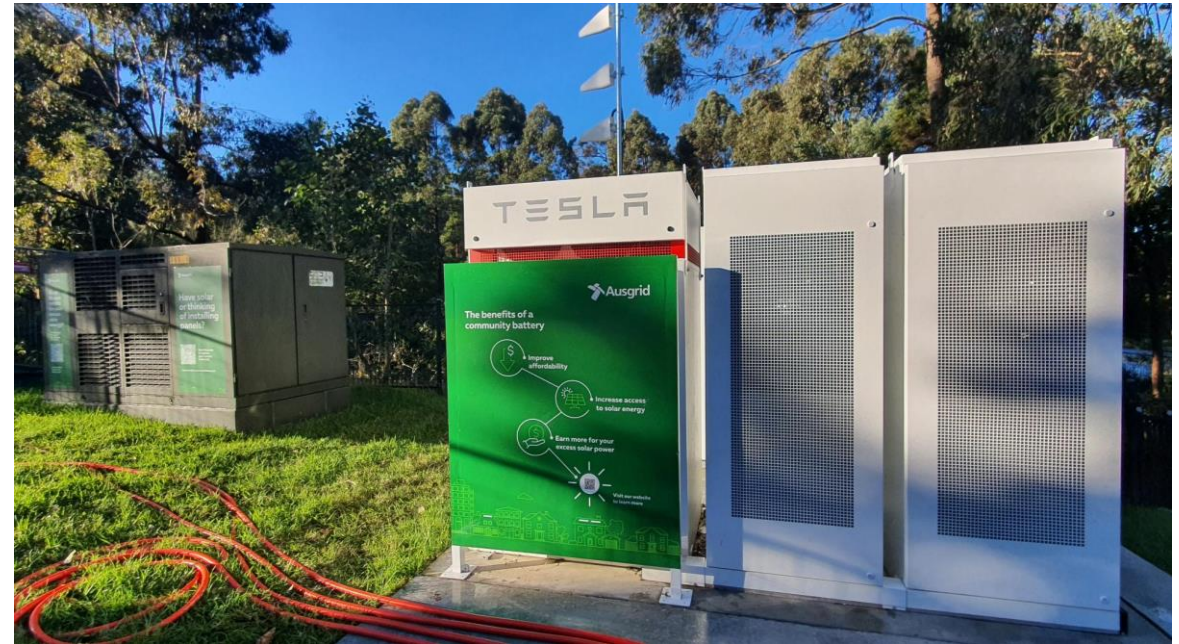
Cameron Park Battery on track to be commissioned 10 June.
