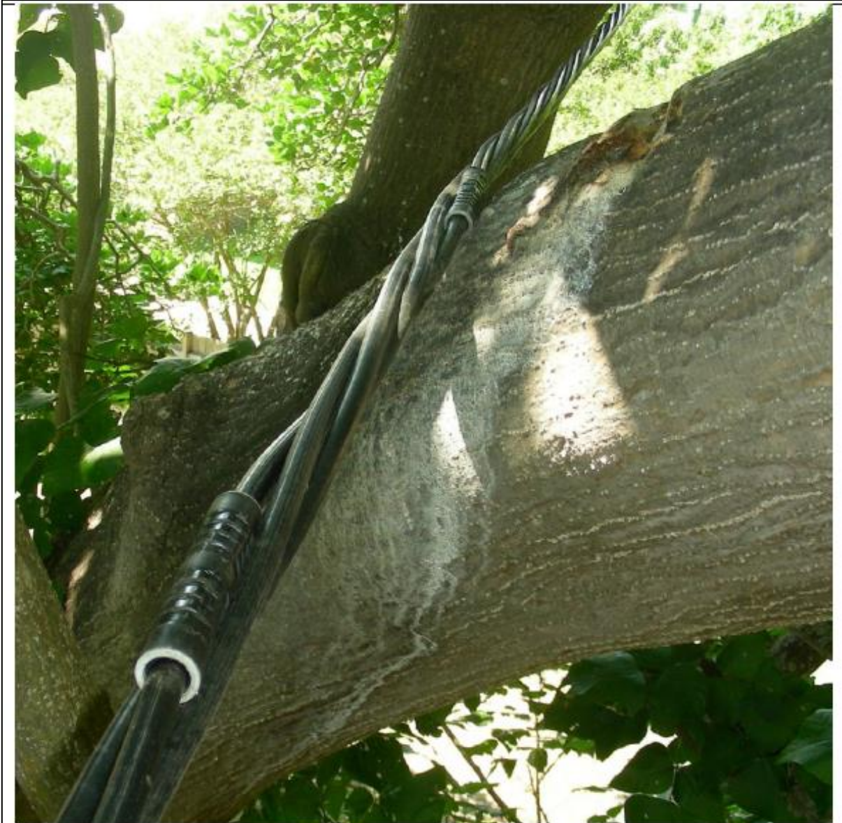
This photo shows damage to a tree branch and the repairs made to an LVABC cable following abrasion (a new piece of cable has been spliced in for the phase that was damaged). The insulation on LVABC is very tough, but can eventually wear through, damaging the cable, the tree, and having potential impacts on safety and reliability.
