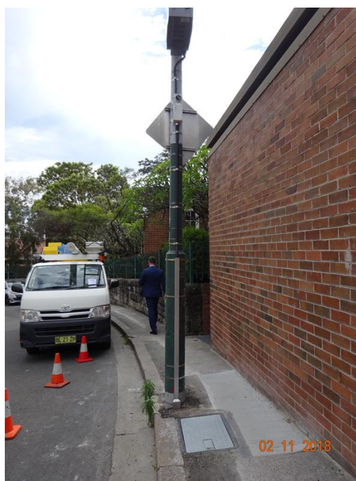
Figure 6: Small Cell antenna installation on steel streetlight standard. Cable installation is external to the pole
