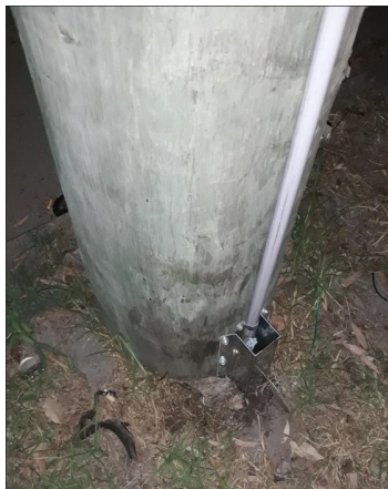
Earthing adjacent to the pole
